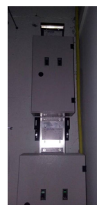
Painéis com Busway Instalado
