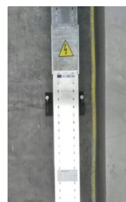
Busway Instalado — Trecho Vertical
